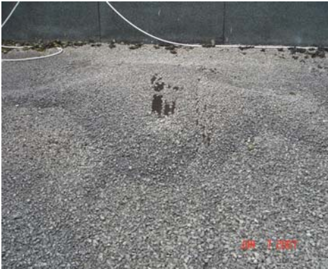
Further Extensive Raised Areas Present
