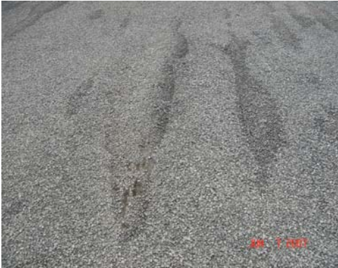
Extensive Raised/Detached Areas Evident
