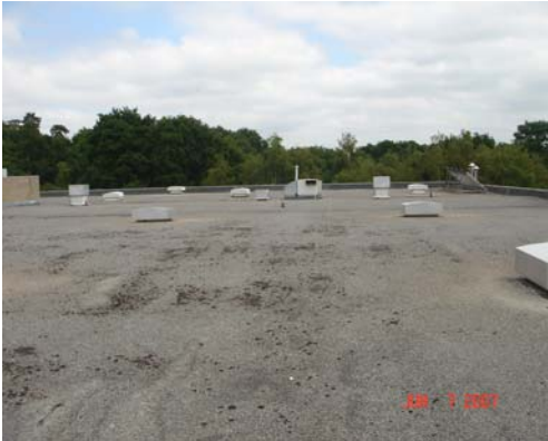
General Overview Highlighting Extensive Defects
