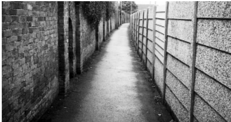
The concrete panelled wall alongside The Tins path badly needs replacement with something more attractive.
